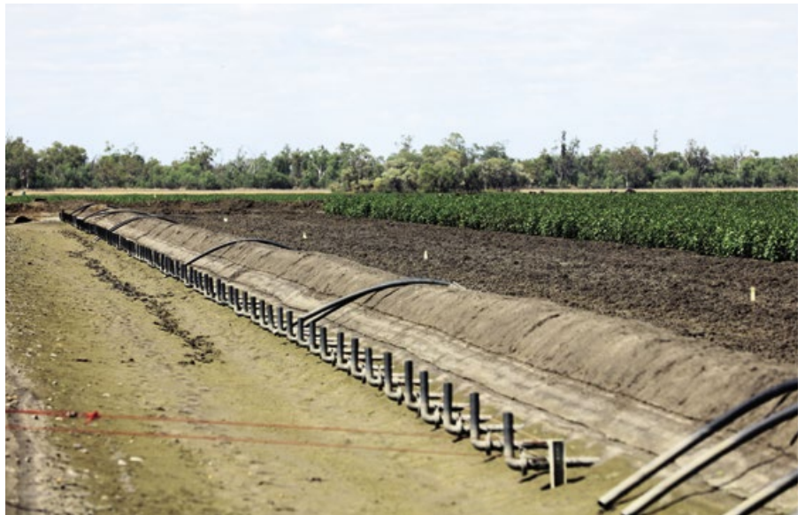
Automation using pipes through the bank in varying configurations is being taken up by growers, with recent analysis showing it makes good sense.
